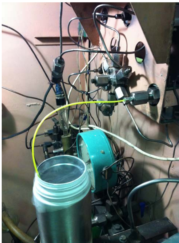
Figure 4. View inside the safety chamber of the high-pressure installation
