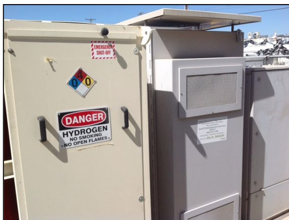
Figure 1. Bulk hydrogen storage containers.
